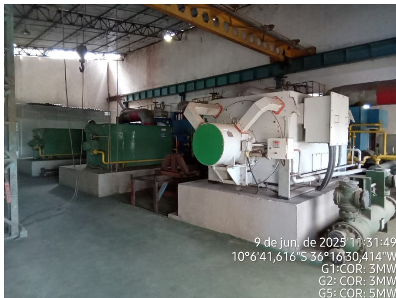
Generators 1, 2, and 5 and their respective turbines (UTE Coruripe Usina COR)
