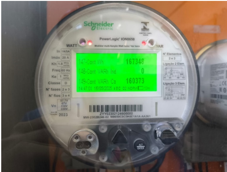
Meter UTE CORURIBE CAMPO FLORIDO - MAIN - MW-2302B246-02
