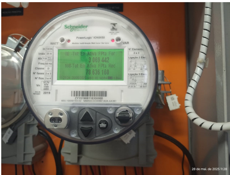
Meter UTE CORURIBE CARNEIRINHO - CHECK - MW-1908B183-02
