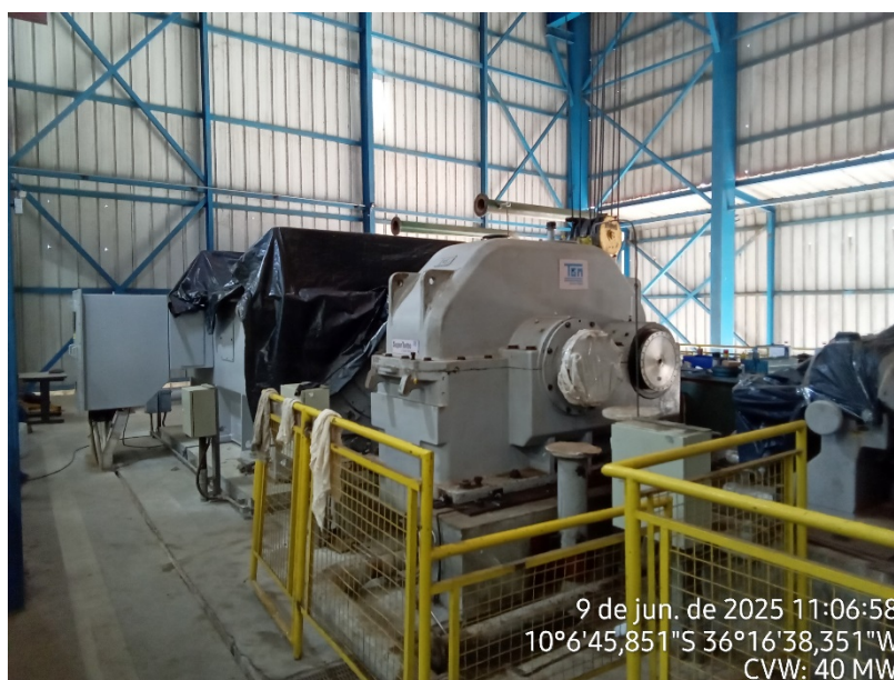
Turbine 6 (Coruripe Energética (CVW))
