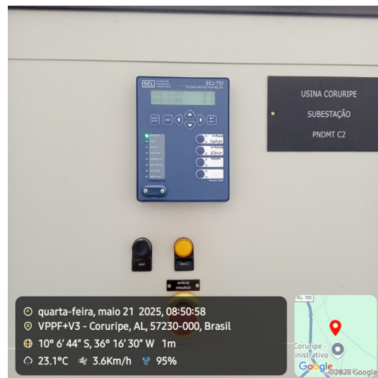
Feeder Protection Relay
