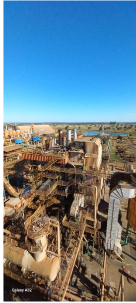
Aerial view of boilers 1 and 2
